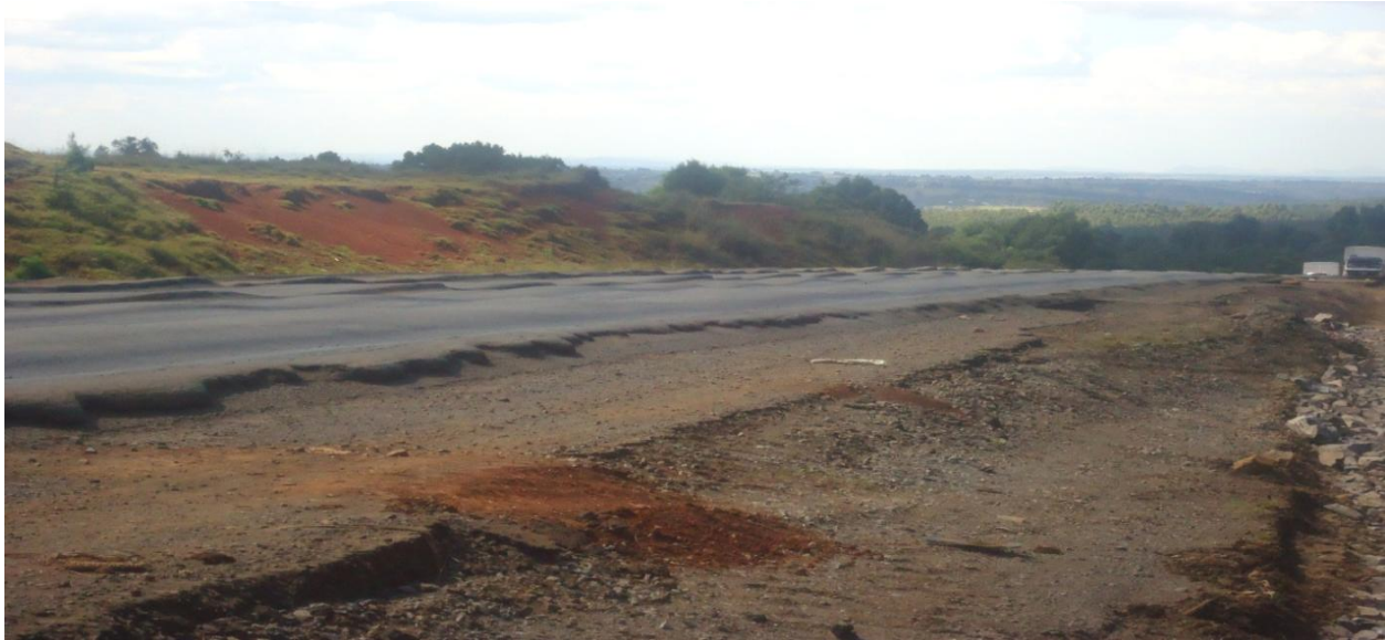
Above: Destruction of road infrastructure between Timboroa and Eldoret caused by overloading.
