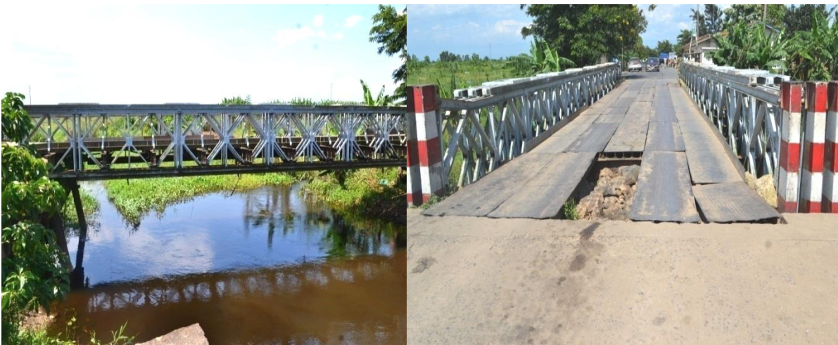
Left: The bridge linking Gatumba-Burundi with Kavimvira-DRC has limited capacity of 50 tons. Right: The Bridge has some damages that require repairs before they escalate.
