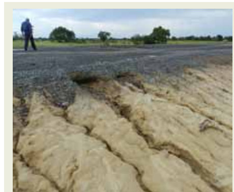
Severe erosion of road side slopes in high rainfall areas.
