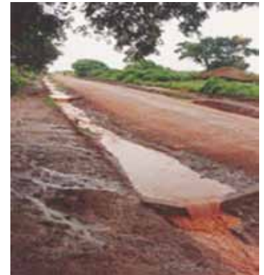
A functioning scour check
