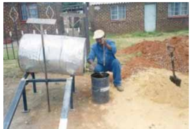
Steel frame stand for decanting emulsion
