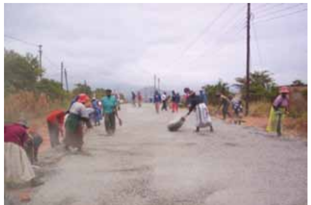
Un-even spreading of aggregate
