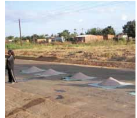
Spotting of aggregate (note the plastic sheet)
