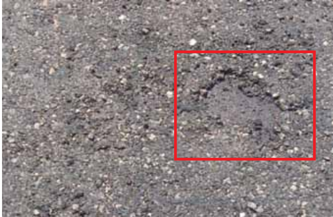
Mark the area of the pothole
