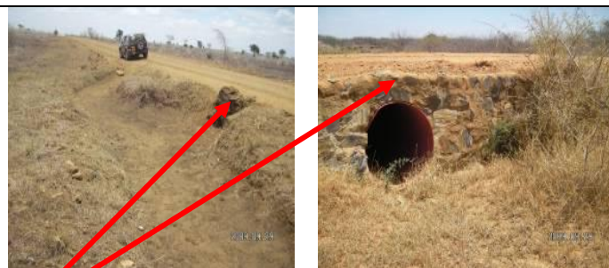
Culverts Lacking headwalls
