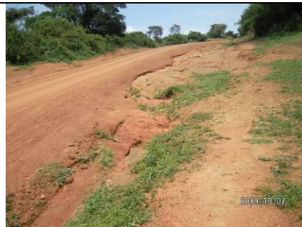
Poor drainage works affecting the road
