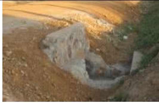
Questionable if headwalls was constructed according to design and specifications
