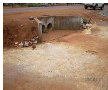
Culvert sections of insufficient size
