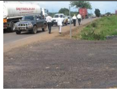
Missing sign and poor surface dressing at Magamaga access
