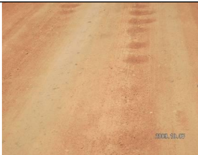
Recently gravelled section failed (poor Camber)
