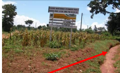
Side drain silted
