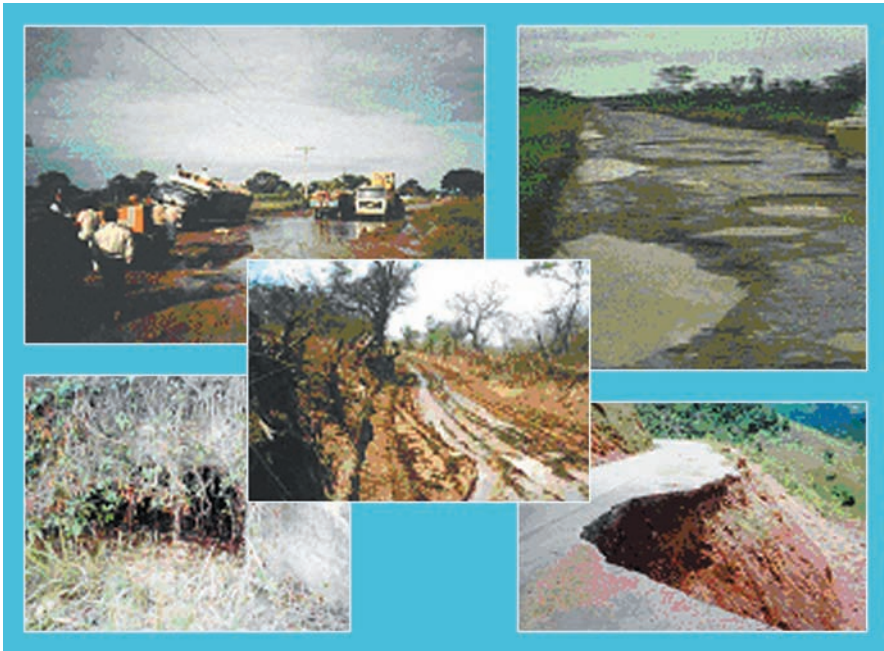
Figure 1. Examples of poor construction and maintenance of roads
